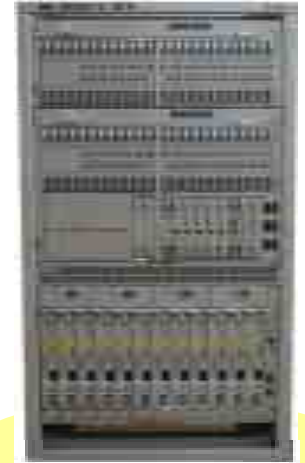
Base Station for NTT DoCoMo
