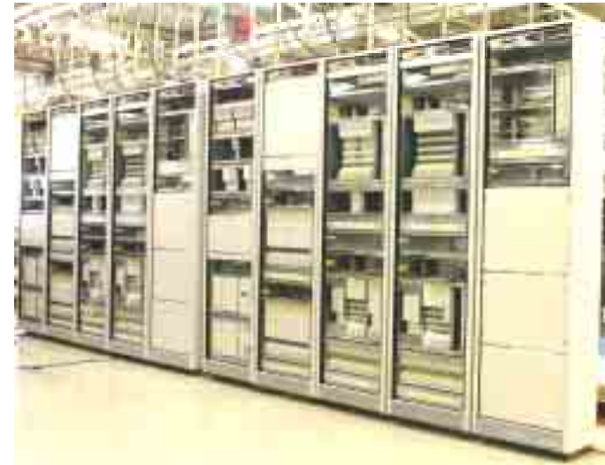
Submarine Line Terminal
